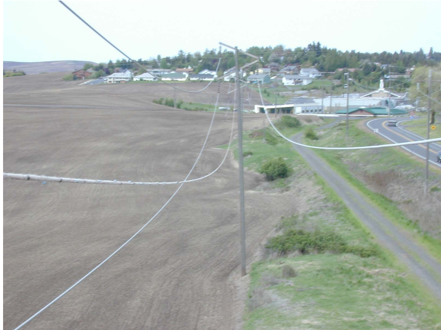
Figure (D.1) 115 kV line with resistive wire installed between the conductors
