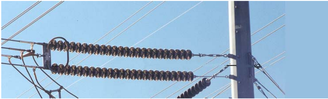
Figure 2. Ceramic Insulators in an Overhead Line
